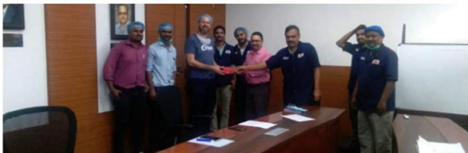
OKA and Vedic team congratulated by Chitale Bandhu team after successful installation and commissioning
